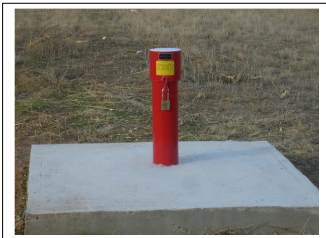
Typical District Monitor Well
